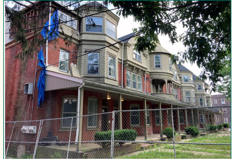
A stretch of apartment buildings on the 800 block of N. Adams Street remains vacant and behind fencing as significant repairs appear to still be needed before the buildings are considered habitable, seen Wednesday, July 5, 2023. William Bretzger/Delaware News Journal
